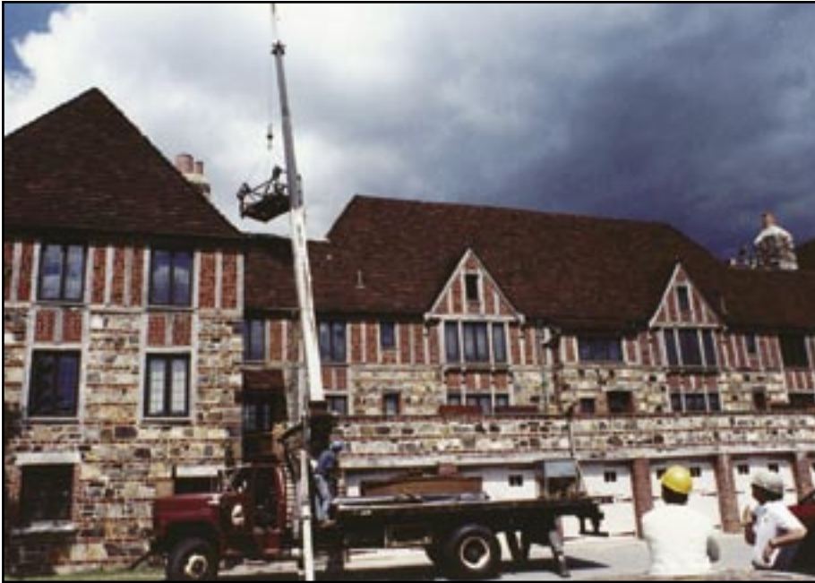
Preparing for a roof inspection of U.S. Naval Officer's Condominiums, Winter Harbor, ME.
